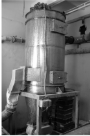
Fig. 5. Combined dust separator of type KP-350-10 introduced into the aspiration system of line No. 1 for production of marshmallow at the Krasnyi Mozyryanin Public Company (Narovlya).
